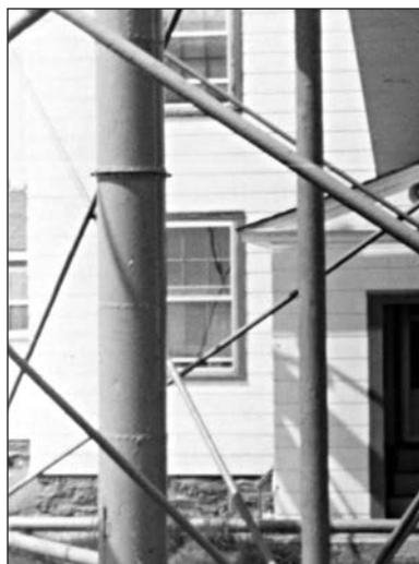
External drop tube of a skeletal tower. Manitou Island, Michigan. U.S. Coast Guard photo.
