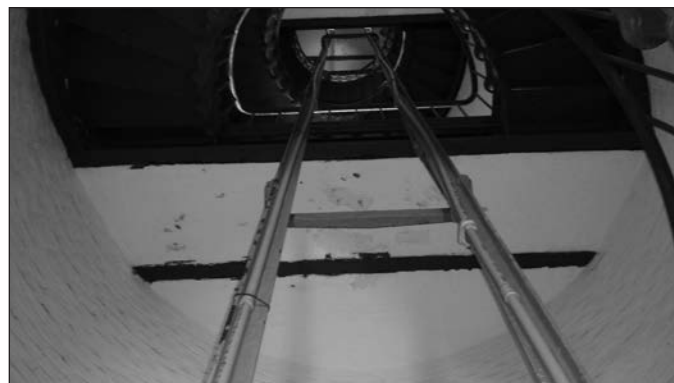
Post 1913 rail system for guiding weights – no longer in use – Cape Hatteras, North Carolina. Photo by Jami Lanier, National Park Service.
