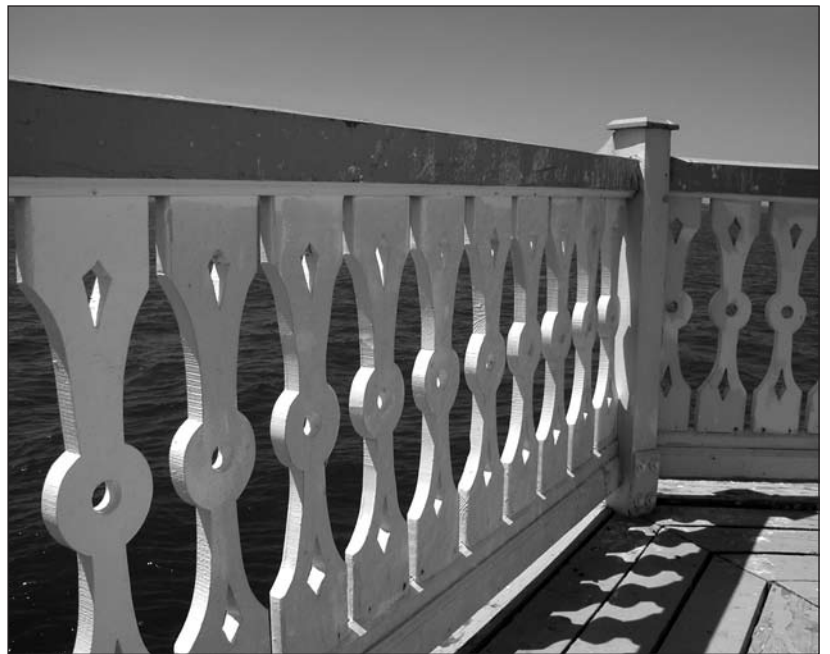
This beautiful railing circles both the main gallery and the lantern room gallery.
