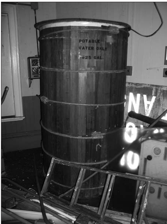
The original 525-gallon cypress water tank is in surprisingly good condition.
