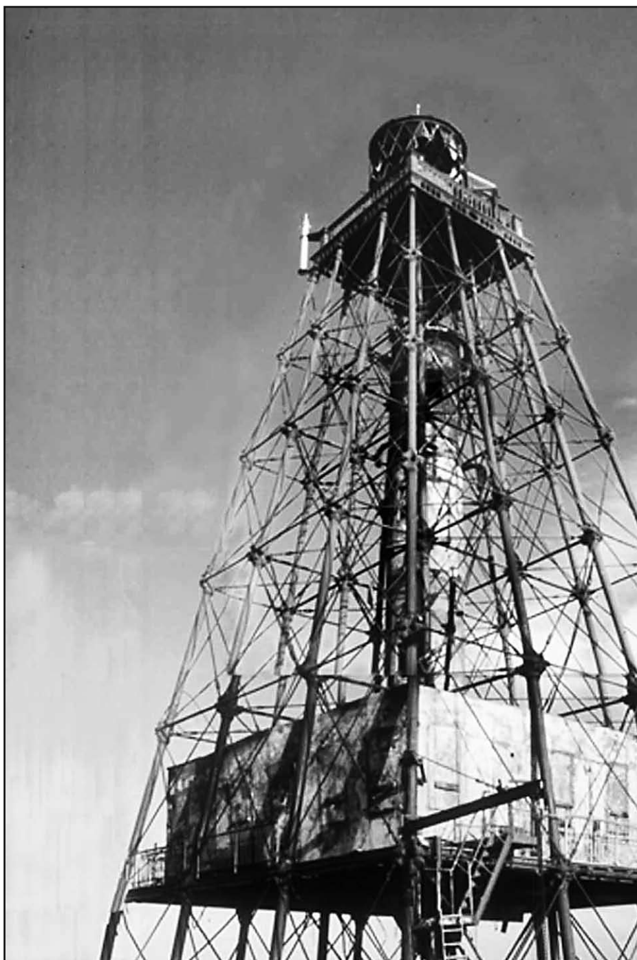
View of the damage to the Sand Key tower. Photo courtesy of the author.
