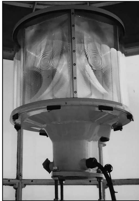
Left – The new Vega optic installed in the lantern room of the Sand Key tower. This new type optic is manufactured in New Zealand and used around the world. Photo courtesy of the author.
