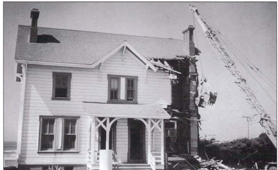
The Coast Guard demolished the original dwelling in 1960 and replaced it with four ranch-style houses. Photo courtesy of Ron Duarte.
