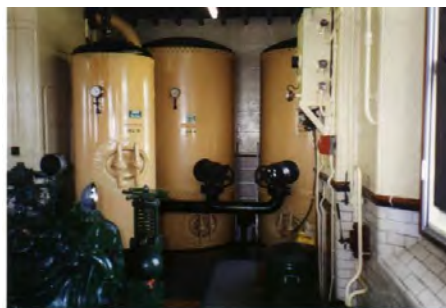
Fig. 5 Air receivers and fog signal equipment
