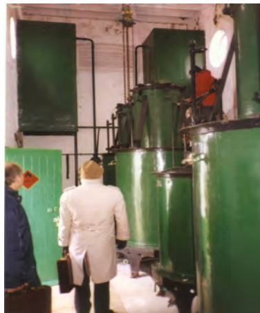
Fig. 10 Moyes equipment, Hurst Point Lighthouse
