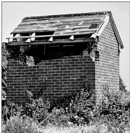
Above – The Cedar Island Light Station oil house prior to restoration. Photo by the author.
