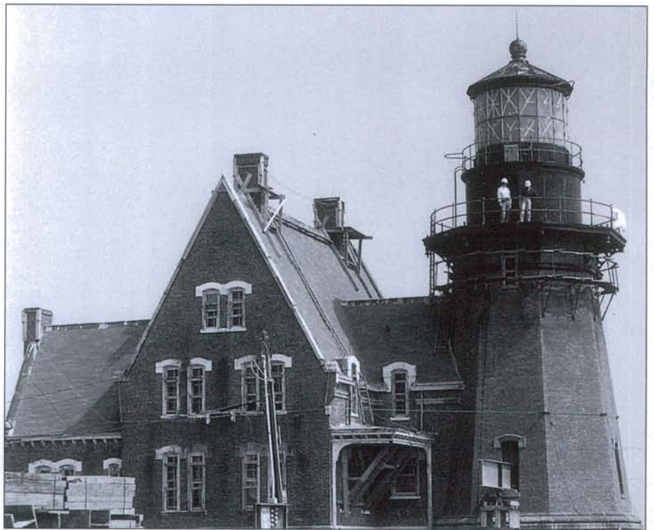
Almost ready to move. Note the extensive bracing around the chimneys, windows and below the upper gallery. An I-beam protrudes out of the lower tower and a steel cable is in place around the entire structure for stability. 1993 photo courtesy of David Richards.
