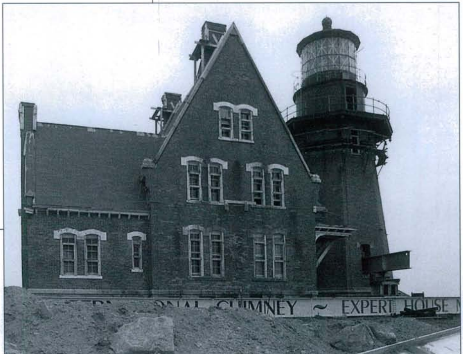
The lighthouse and dwellings ready to move. Note the huge I-beam protruding from the lower window in the tower. The dwelling windows have all been heavily braced with wood frames and cross pieces and the lantern room glass panes are taped. Photo taken August 13, 1993 by Joe Lebherz.
